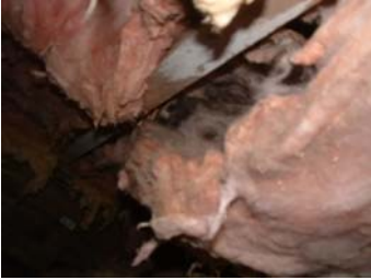
Photo 4 – No Wire Lacing (Moisture)
