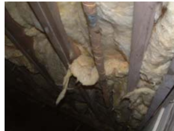
Photo 30 – No Insulation in Bay
