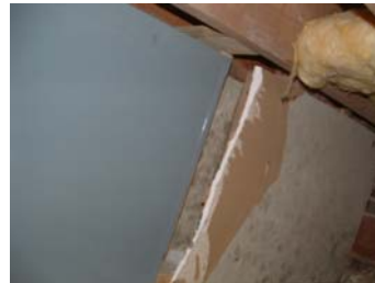
Photo 36 – Breach in Firewall
