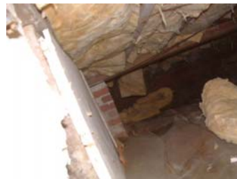
Photo 37 – Breach in Firewall/Debris/Single Layer Batts
