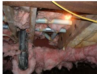
Photo 2 – Missing Insulation @ Bay
