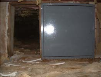
Photo 21 – Void @ Improperly Installed Fire Door
