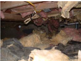
Photo 6 – Debris and Single Batted Bays
