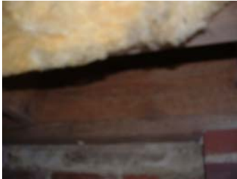
Photo 31 – No Insulation in Joist Bay
