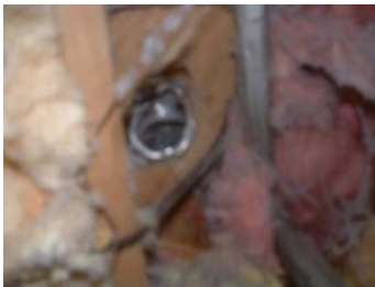
Photo 43 – Missing Duct Work
