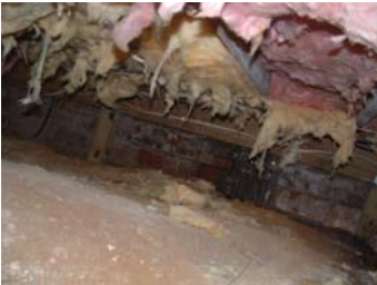
Photo 5 – Moisture Penetration – Poor Installation
