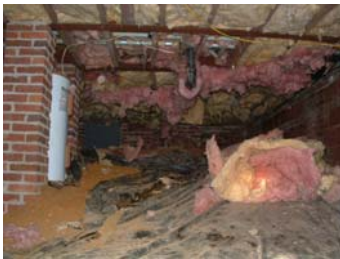
Photo 1 – Uninsulated Water Heater/Pipes
