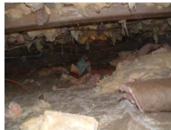
Photo 18 – Single Layer Batts and Debris
