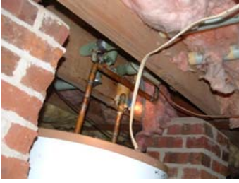
Photo 3 – Missing Insulation @ Bay
