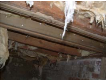
Photo 57 – No Insulation in Joist Bays
