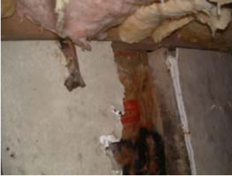
Photo 38 – Moisture/Breach in Wall
