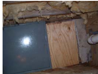
Photo 19 – Improperly Installed Fire Door/Breach in Wall
