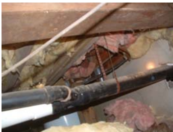
Photo 15 – No Insulation in Bay
