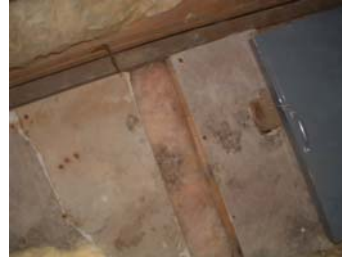
Photo 63 – Moisture/Breach in Firewall
