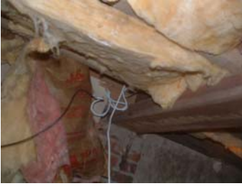
Photo 49 – No Wire Ties/Cable Wires
