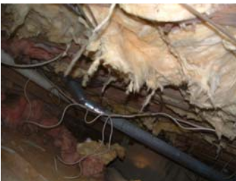
Photo 23 – Single Battis/Improperly Secured Electric Wires
