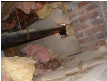
Photo 16 – Missing Insulation in Bay – Breach in Firewall
