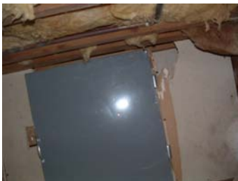
Photo 33 – Breach in Firewall
