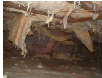
Photo 46 – No Wire Lacing
