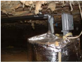
Photo 14 – Insulated Water Heater
