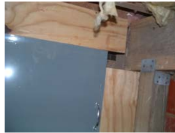
Photo 17 – Improperly Installed Access Door
