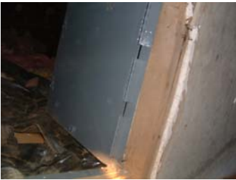
Photo 12 – Improperly Installed Access Panel
