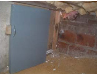
Photo 51 – Moisture/Breach in Firewall
