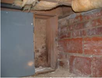
Photo 39 – Moisture/Breach in Wall
