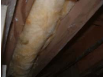
Photo 62 – No Insulation in Joist Bays
