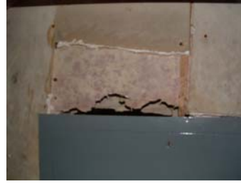
Photo 7 – Breach at Firewall
