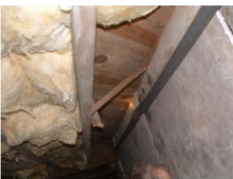
Photo 41 – No Insulation in Joist Bay
