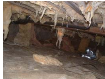
Photo 60 – No Wire Lacings
