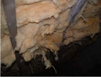
Photo 20 – Lack of Wire Lacing
