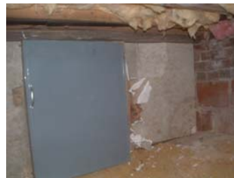
Photo 48 – Breach at Firewall
