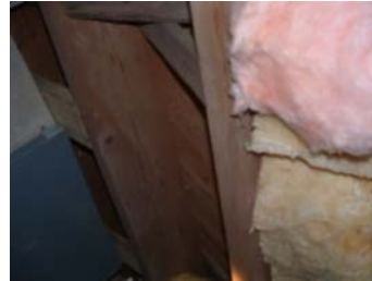
Photo 35 – No Insulation in Bay
