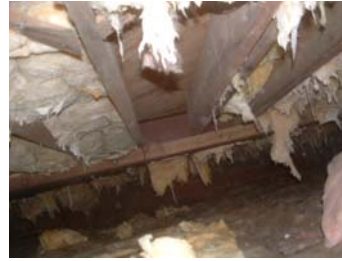
Photo 58 – No Insulation in Joist Bays
