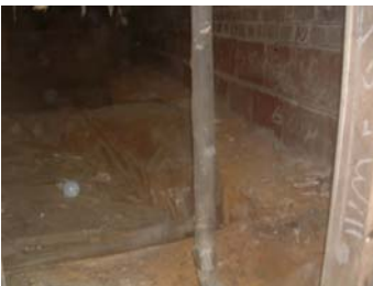
Photo 52 – Access Panel Centers Pipe – Hard to Enter
