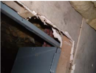
Photo 13 – Breach at Firewall
