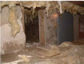
Photo 56 – Moisture/Breaches in Firewall
