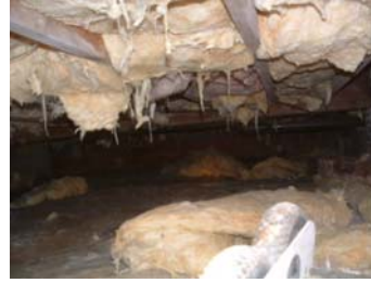
Photo 42 – Debris/Lack of Wire Lacing
