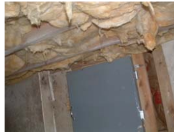
Photo 29 – Voids in Firewall
