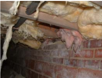
Photo 40 – No Insulation in Joist Bay
