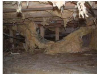
Photo 59 – No Wire Lacings
