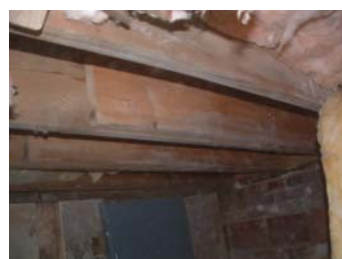
Photo 61 – No Insulation in Joist Bays
