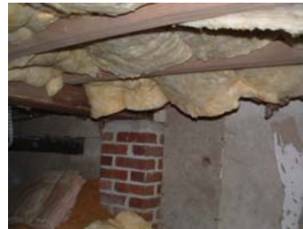
Photo 10 – Missing Wire Ties/Party Wall Breach
