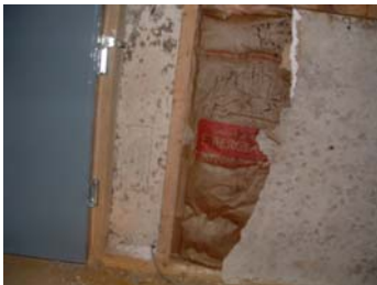
Photo 27 – Breach in Firewall
