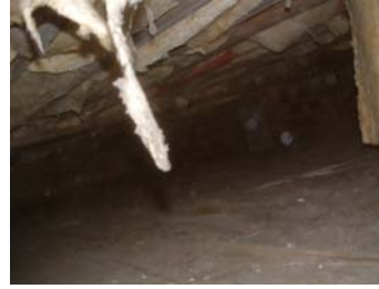
Photo 53 – Missing Wire Lacings
