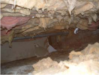
Photo 50 – Breach in Firewall
