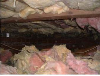
Photo 11 – Debris/Improperly Installed Access Panel
